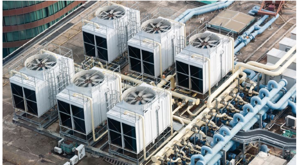
Building systems are being designed with 50% more electrical capacity and 30% more heating and cooling capacity than is ever needed.
