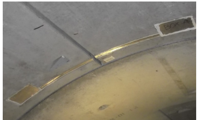
The Fibre Optic Monitoring Technology
