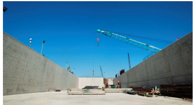
Deephams Sewage Treatment Inlet Works
